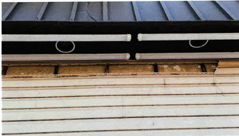
Broken vinyl siding and exposed wood framing.
