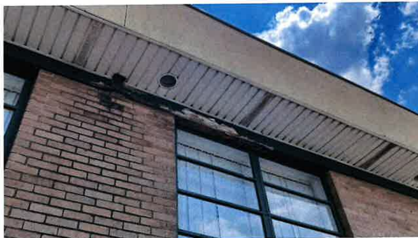
Exposed wood soffit/facia and disconnected downspout.
