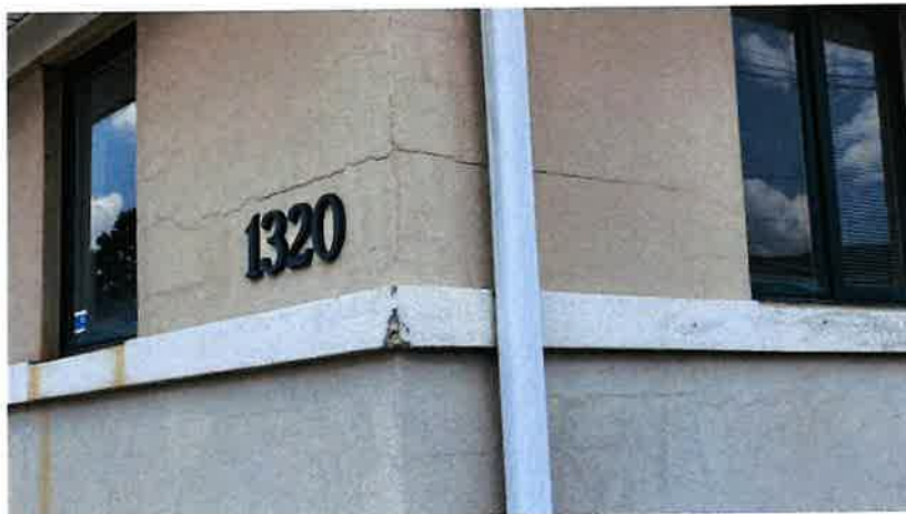
Cracks in exterior wall
