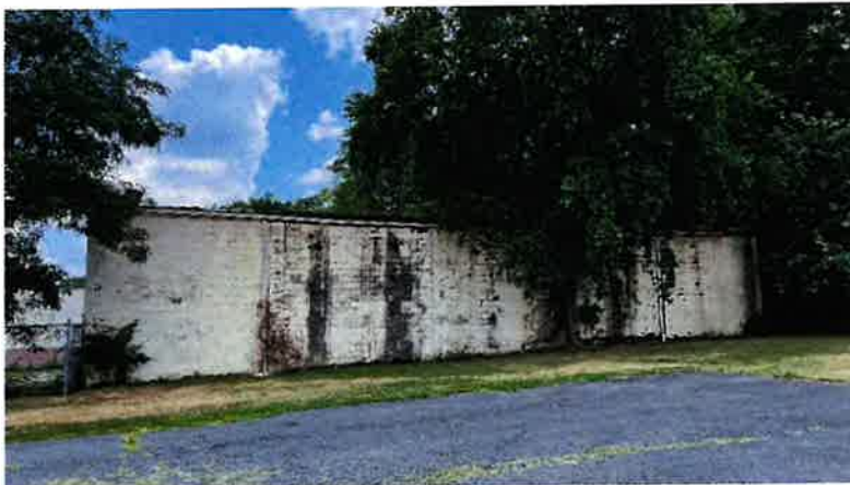
Dilapidated structure and roof from side yard.
