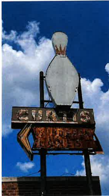
Rusted and deteriorating signage
