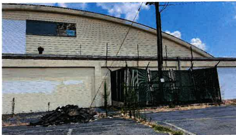
Haphazard loose building debris in rear
