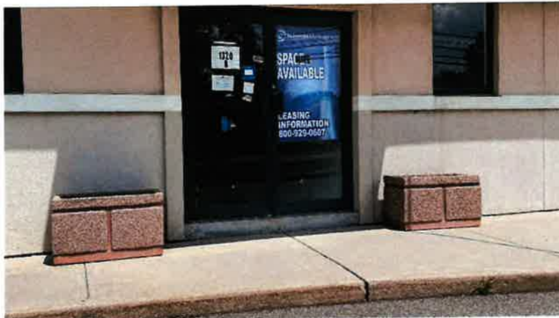
ADA non-compliant front entry on Parkway Ave.
