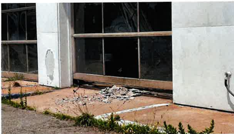
Broken window, loose building material, and exposure of building interior.
