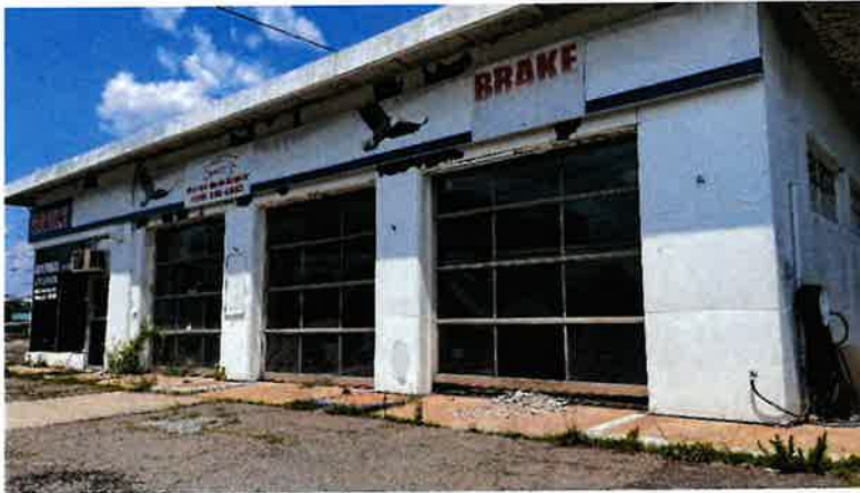
Dilapidated garage bays
